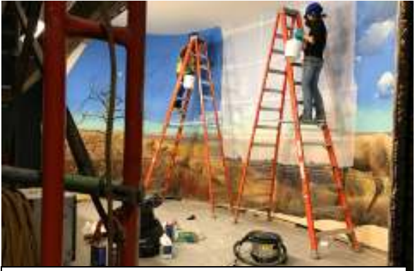
Crews cleaned the old diorama paintings before they put in the foreground.
